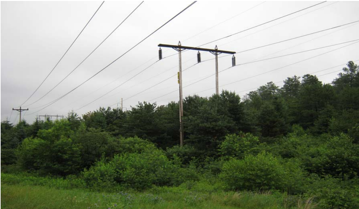
Figure V-11 - Northeast view of PSNH 115kV circuit P145 with circuit V182 shown in the background. (Photo by NEI)
