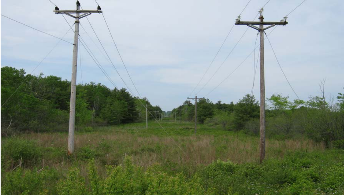
Figure V-9 - Example of 34.5 kV Unitil sub-transmission line ROW. (Photo by NEI)
