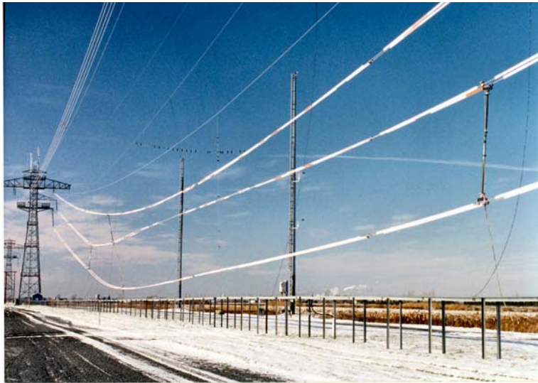
Figure F-9-Excessive sag as a result of galloping. (Photo courtesy of CIGRE)
