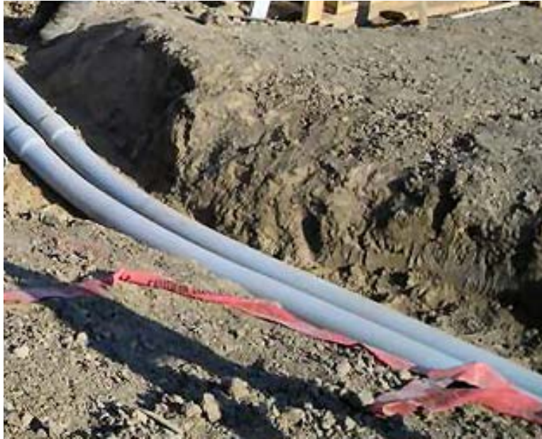
Figure B-5 - Conduit and Trench for Underground Distribution (Photo by NEI-Grand Prairie, Alberta)
