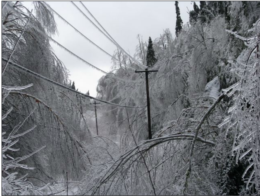
Figure I-2 – Damage in PSNH distribution line corridor. (Photo courtesy of PSNH. Exact location unknown.)
