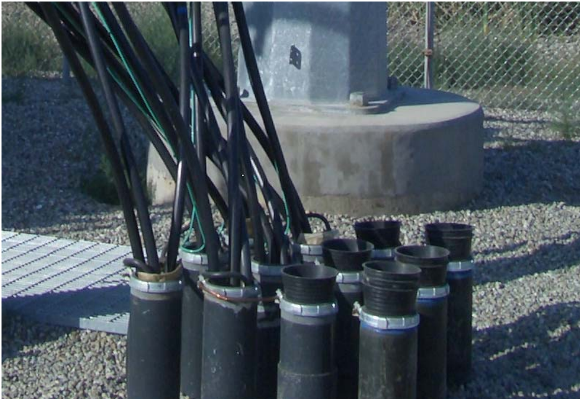
Figure B-3 – Typical underground conduit and cable. (Photo by NEI)
