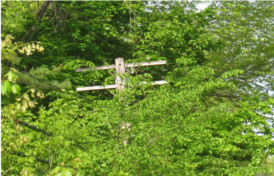
Figure V-14 – NESC Rule 218 violation in Unutil service area. (Photo by NEI)
