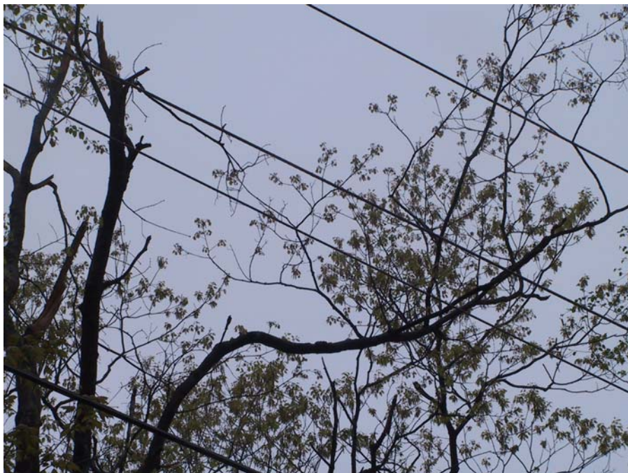
Figure V-5 - Small diameter immature trees broken above conductors in New Ipswich, NH. (Photo by NEI)
