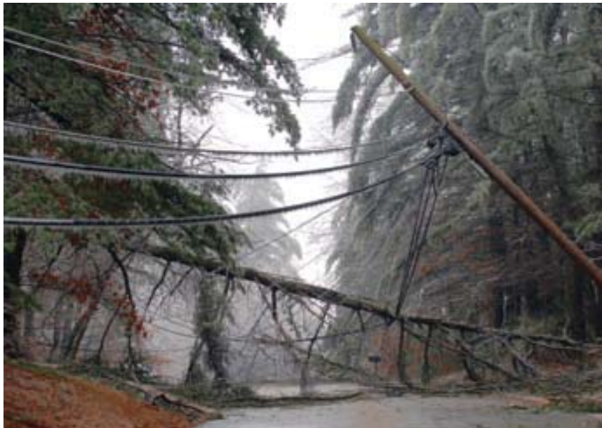
Figure I-3 - Impassable roads due to ice damage in Londonderry, NH (Photo courtesy of PSNH)
